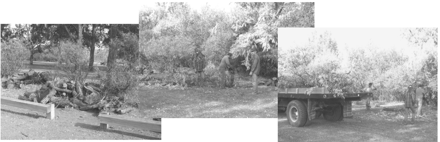
RO removal at Sanford Park; The project was completed by DugRign Tree Trimming and B & S Tree Trimming services.
